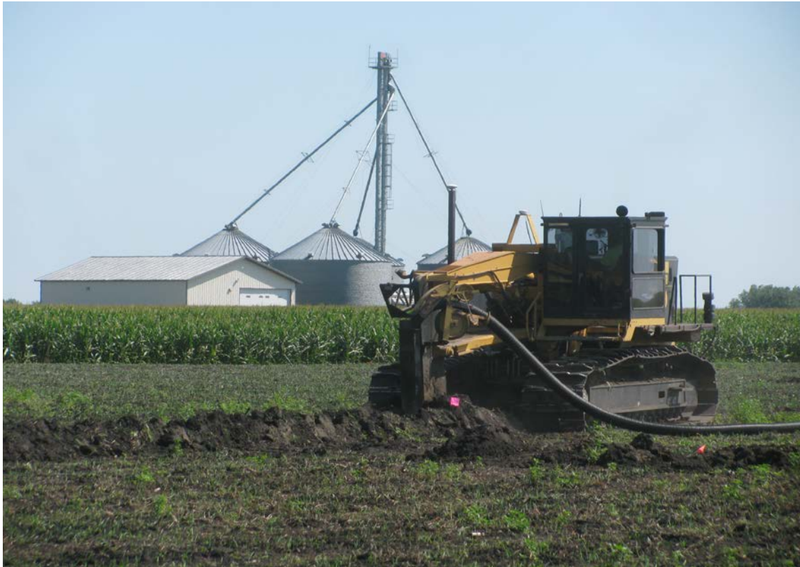
Figure 4 - One of the benefits of the Prevented Planting claims and cover crops is the ability to install drainage tile this summer.
