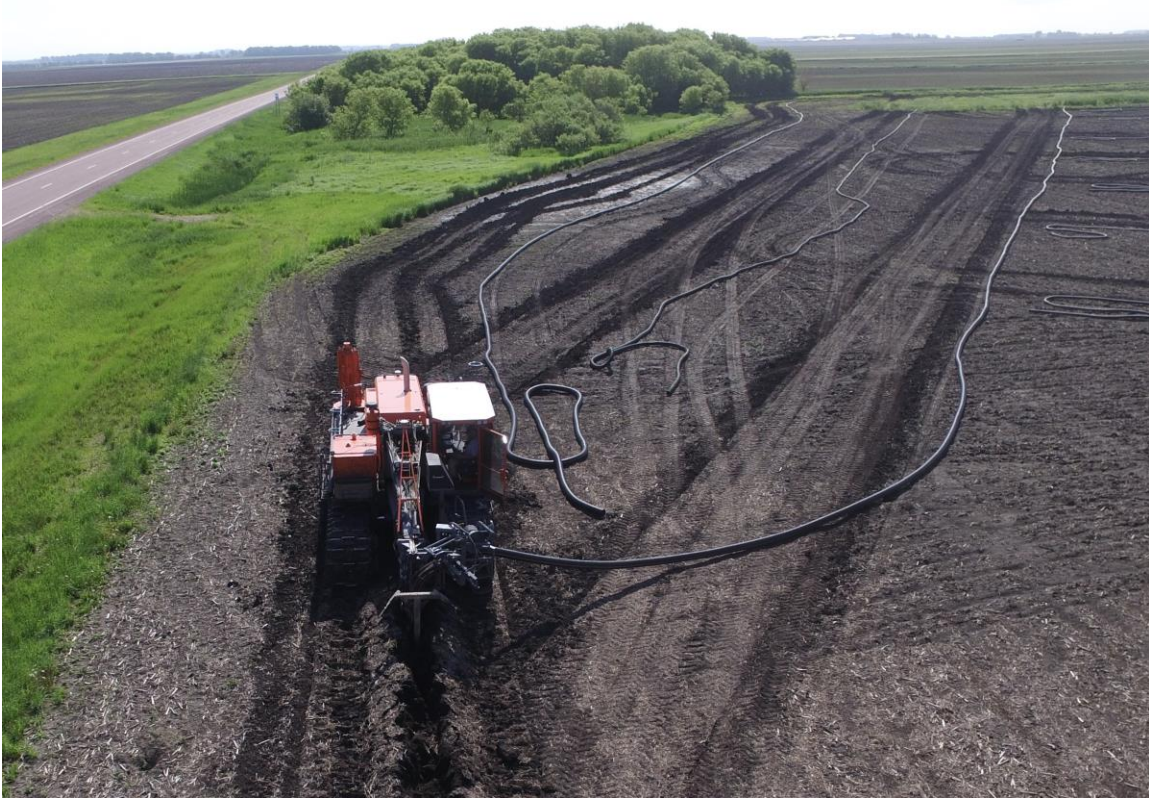
Figure 4 - This is a picture of a tile plow installing plastic tile through a wet area. Given the weather patterns that we have experienced the past couple of years, having adequate drainage tile is becoming more and more critical. Farms with good drainage produce the best crops. Tile is the most important investment landowners can make in their farmland.
